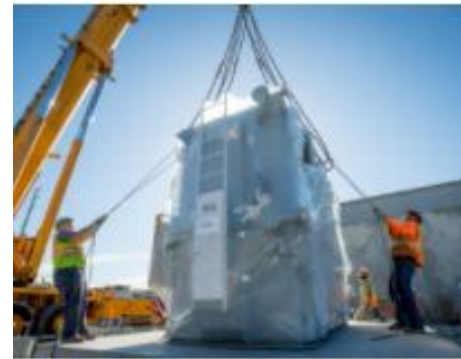
Traction Power Facilities
