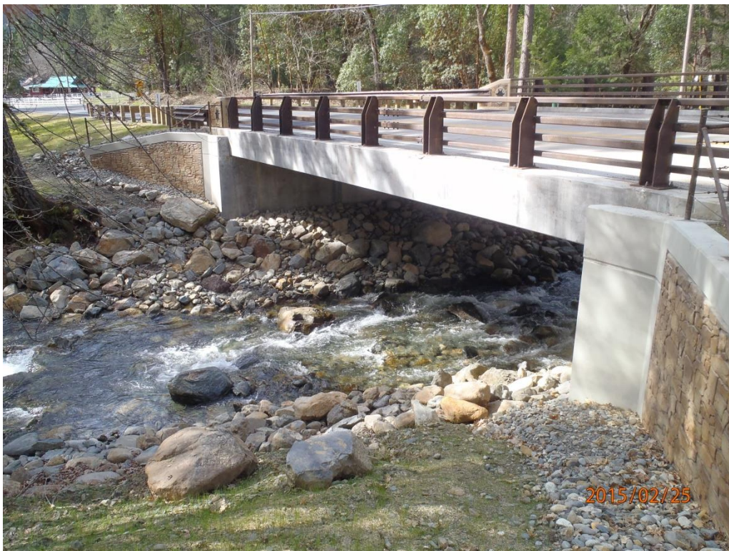
*Fort Goff (District 2, Redding) Fish Passage structure
