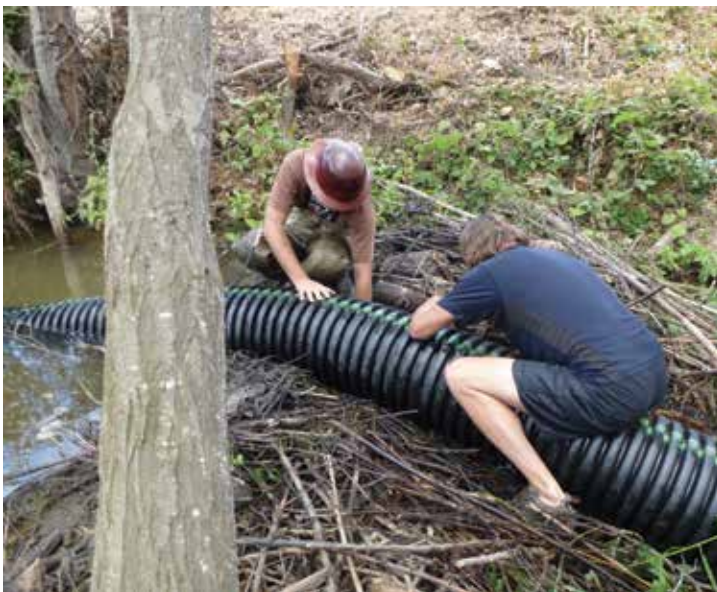
Kevin Swift (on right) of Swift Water Design installs flow control device for Caltrans in Monterey County. (Photo: Kate Lundquist/OAEC)
