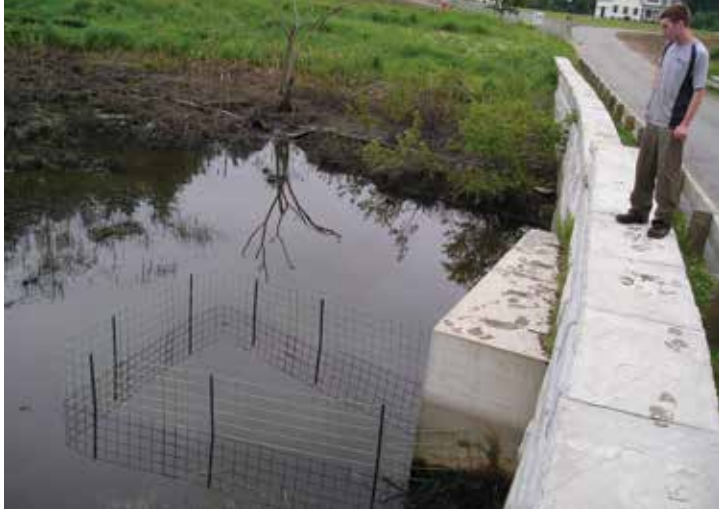
Trapezoidal protection fence in Westford, MA prevents beaver from blocking the culvert. (Photo: Mike Callahan/Beaver Solutions, LLC)
