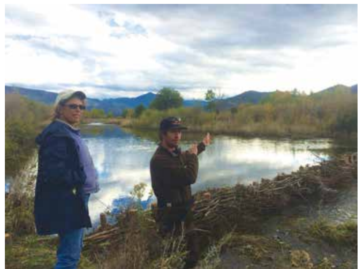
Betsy Stapleton and Peter Thamer standing near a newly installed beaver dam analogue on the Scott River. (Photo: Scott River Watershed Council)
